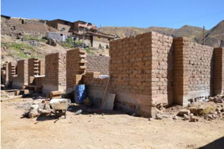
Windows removed and cracked blocks replaced, the school is ready for the geomesh. Courtesy of GHI/Stanford/PUCP
